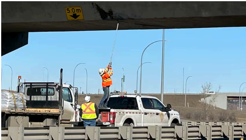
Canadian Pacific Kansas City structural engineers examine the railway bridge above Circle Drive, south of the Attridge Drive overpass, on Monday, a day after a vehicle struck it. (Phil Tank/CBC)
