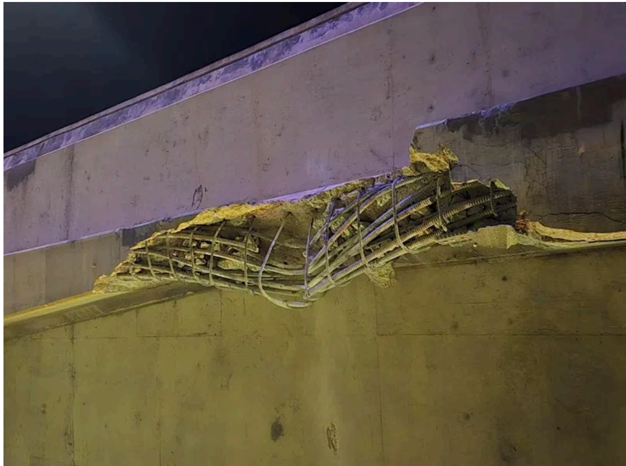
City crews are now working to repair the damaged section of the overpass (Photos courtesy City of Saskatoon)
