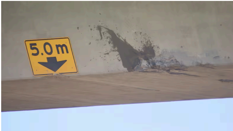
Damage underneath the railway overpass above Circle Drive is visible next to the sign indicating the clearance under the overpass is five metres. (Chanss Lagaden/CBC)
