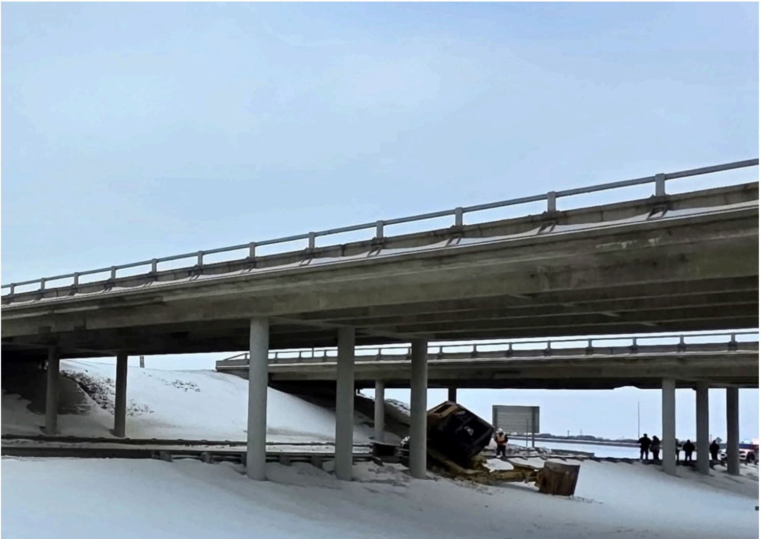
The other half of the excavator that hit the overpass. | Jon Perez
